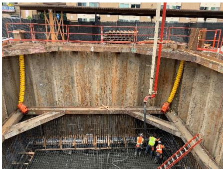
San Lorenzo Sewer Lift Station
