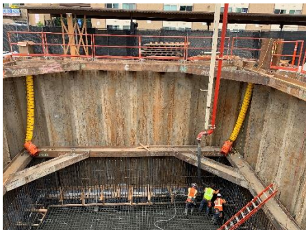
San Lorenzo Sewer Lift Station
