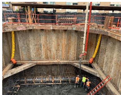
San Lorenzo Sewer Lift Station
