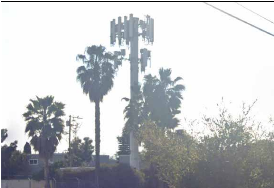
2120 South Bristol Street – Co-location
