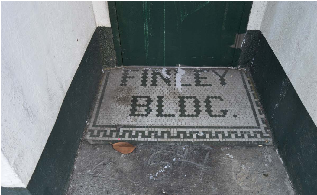
Detail of ceramic tile threshold at original hotel entrance, view facing south.
